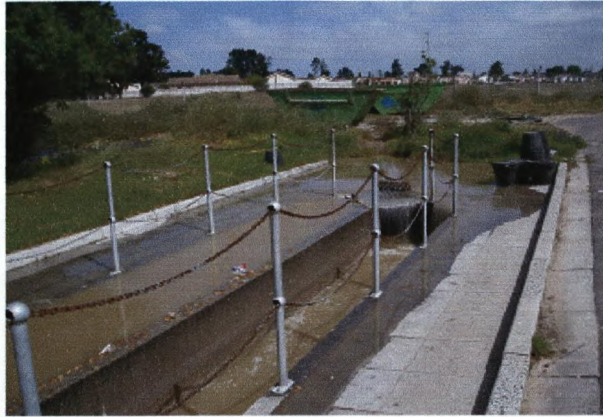
I. Input (Raw wastewater flows into the Scottsdene WWTW)
