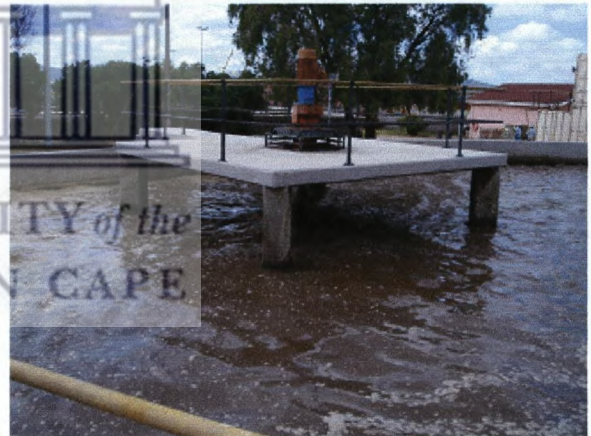
IV. Anoxic pond (Removal of nitrogen by microorganisms to optimize the operation conditions)
