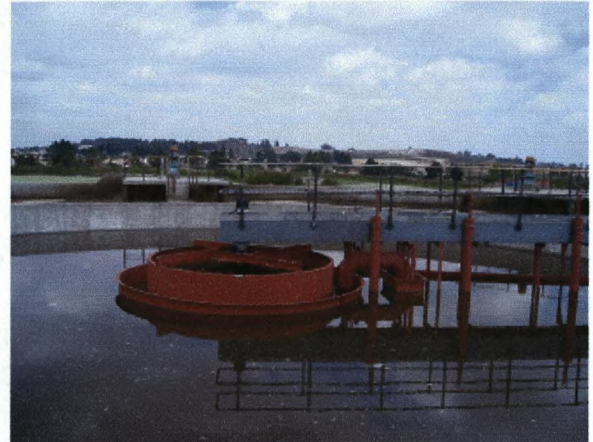
VI. Maturation pond (further purification of the relatively clean wastewater takes place)
