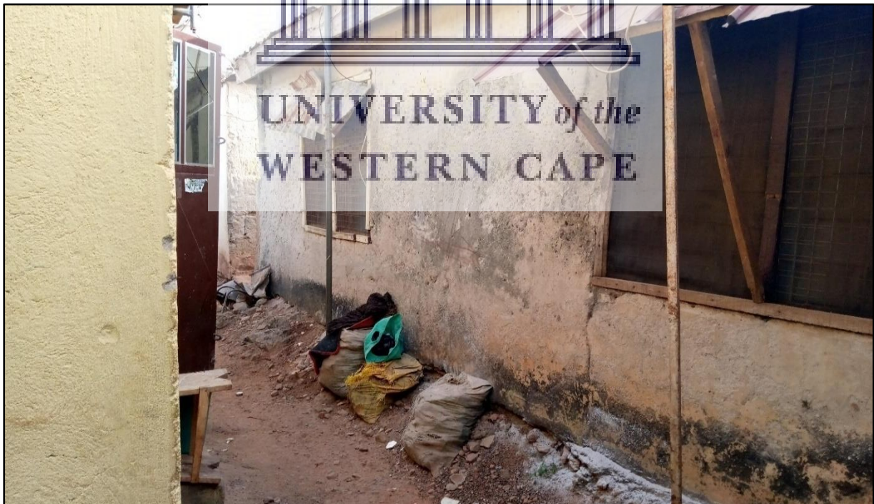
Figure 9: State of houses in old residential area in Aburaso Source (Fieldwork, 2020)
