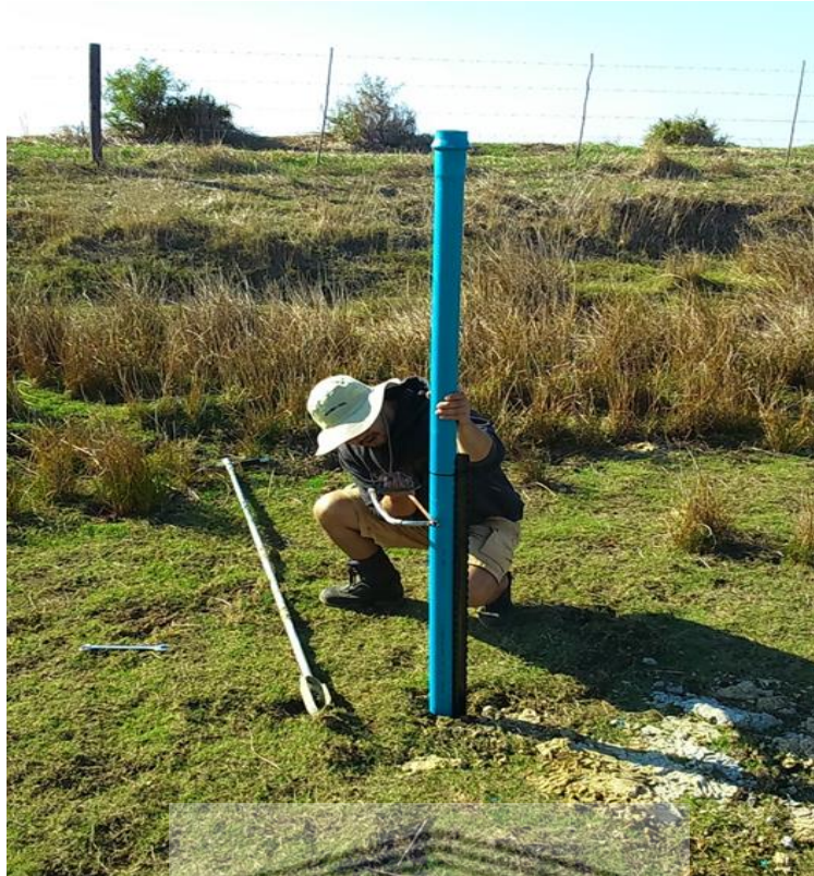
Figure 3.11 Installation of the PVC pipe into which the OTT water level logger was placed on the Lower Kars River at Zeekoevlei farm
