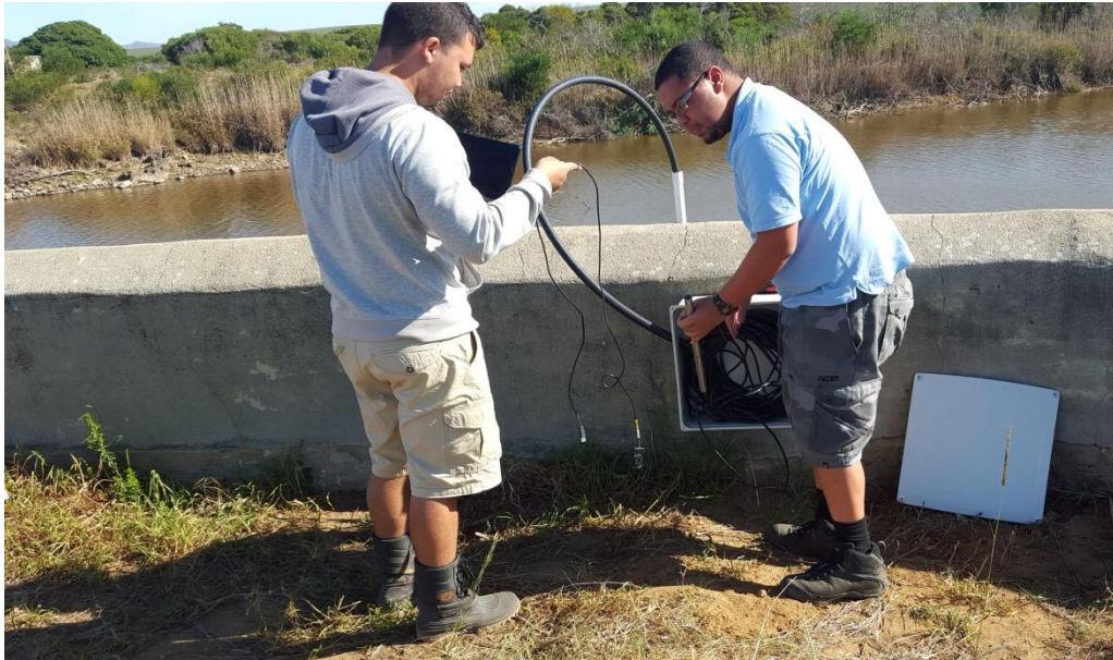
Figure 3.9 The housing box for the data logger download port fixed to the weir wall
