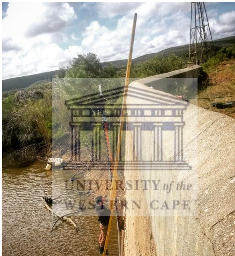
Figure 3.8 Installation of the OTT water level logger which was attached to a gauge plate on the side wall of the weir at Nacht Wacht farm
