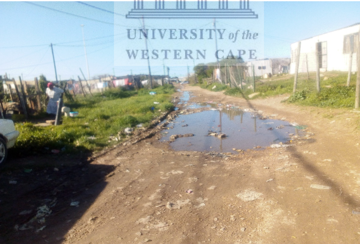
7. Running water from and caused by a leaking tap
