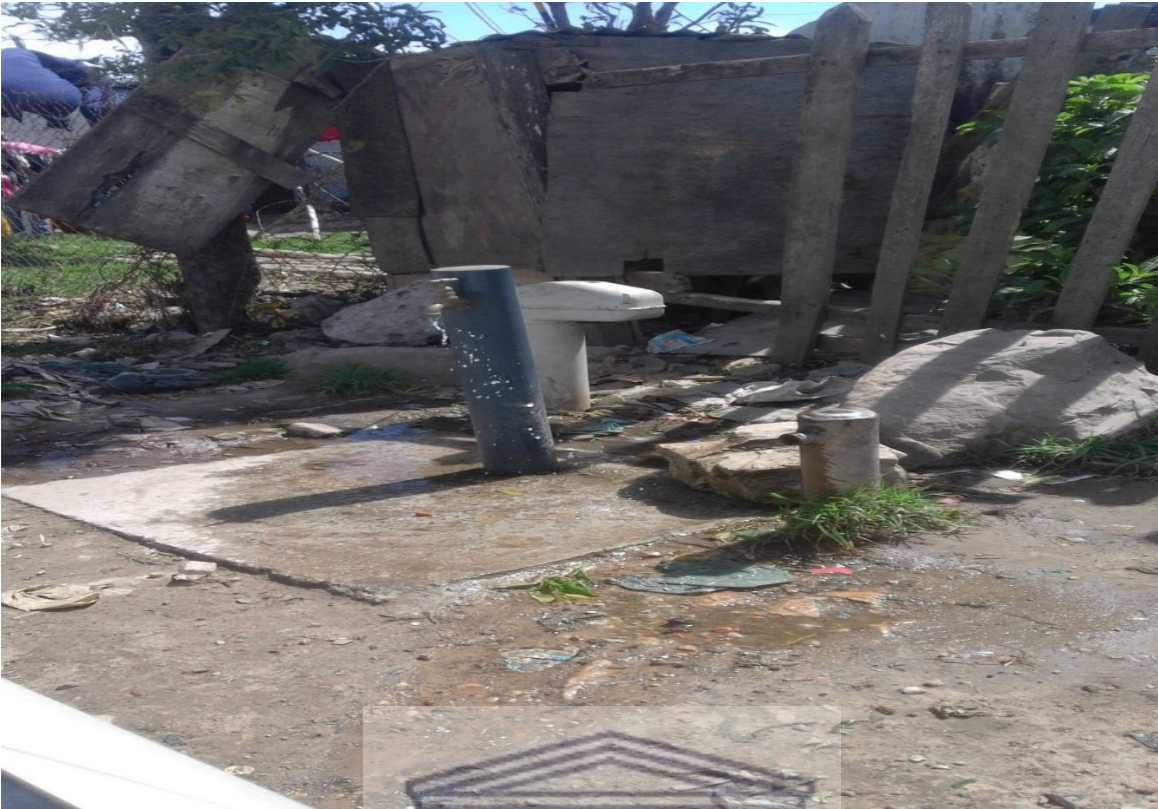
6. A leaking tap
