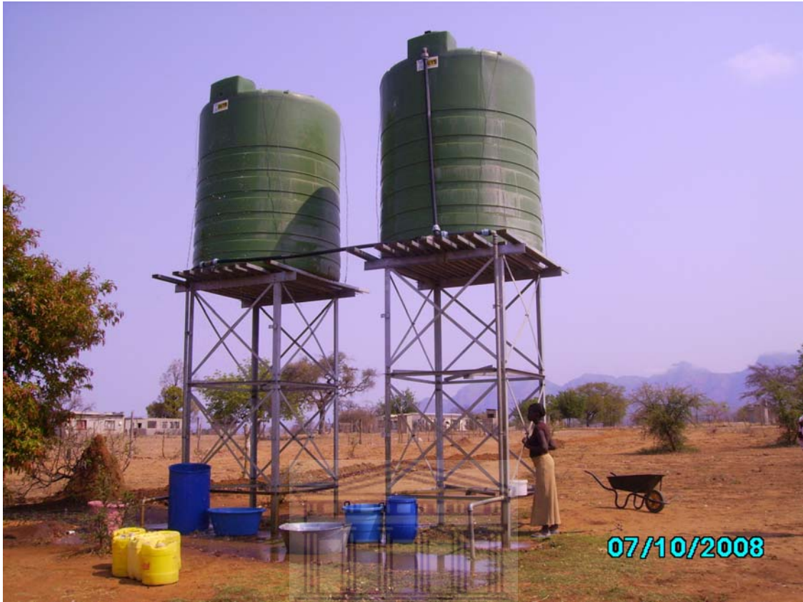
Insert/plate 5.7: Jojo tanks for communal water supply in Worcester. The tanks are owned and managed by the Maruleng local municipality and the DWA regional offices at the Oaks.
