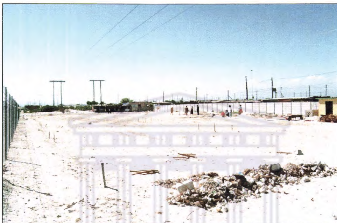
Figure 3: SCAGA garden underneath powerlines. Initial stage: fences and sheds were erected, ground ripped, pump installed and the vegetable plots demarcated.
