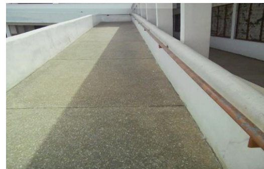
Figure 5. 39: A ramp with only one handrail at one of the university libraries, UL1 (Source: Field data, 2022)
