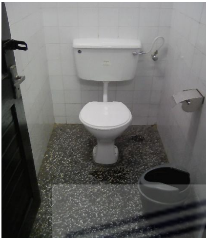
Figure 5. 48: A washroom not disability friendly in one of the university libraries (UL1) (Source: Field data, 2022)
